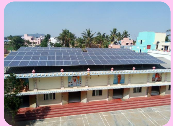
SOLAR PANEL FACILITY
